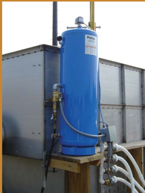
Air Scour Air Reservoir Added Spring 2007
